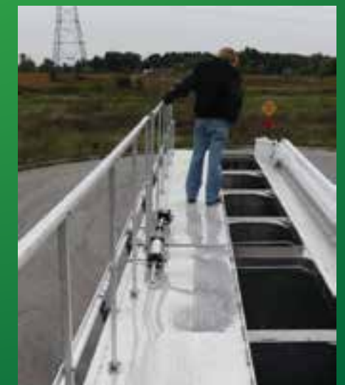
Air operated hand rail on the catwalk.
